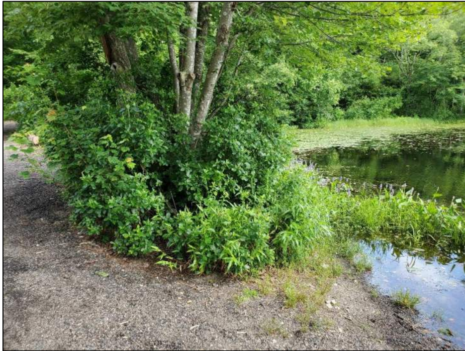
Photo No. 5. Upstream slope from STA 2+20 looking right. Note the trees up to 10 inches in diameter growing through the upstream slope.
