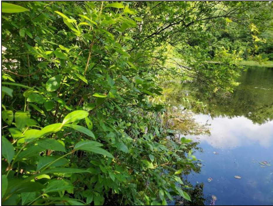
Photo No. 1. Upstream slope from STA 1+20 looking right. Note the dense woody vegetation growing on the upstream slope.
