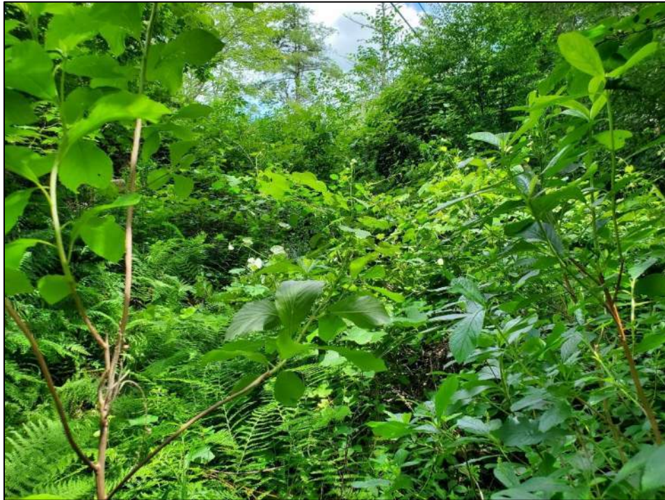
Photo No. 17. Downstream slope at STA 2+50 looking right. Note the dense vegetation and woody brush.
