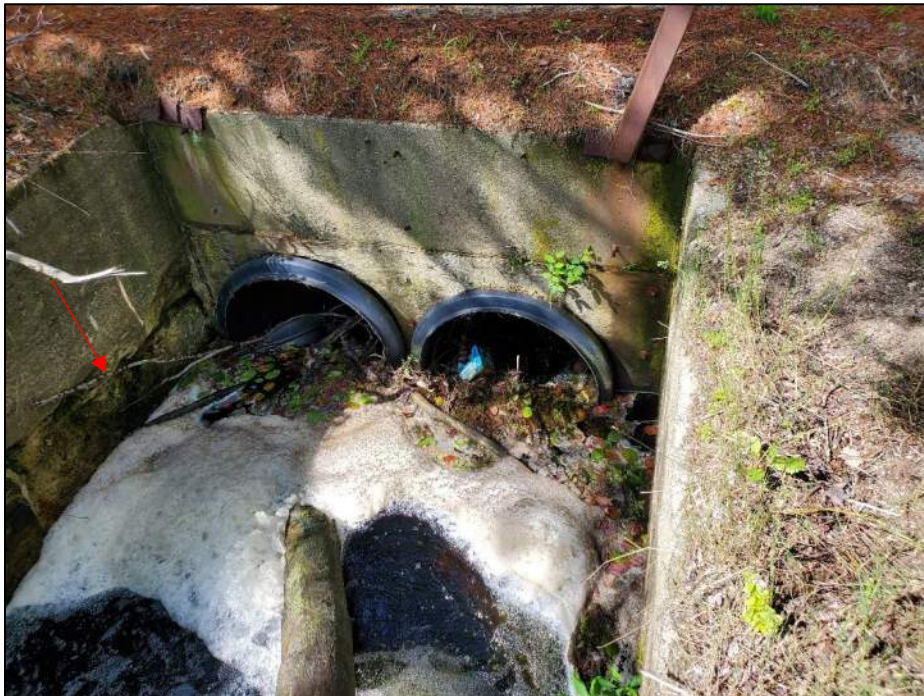
Photo No. 22. Spillway stilling basin and spillway culvert inlets. Note the vegetation and garbage choking the culvert intakes. Note the spall in the stilling basin left wall (arrow).
