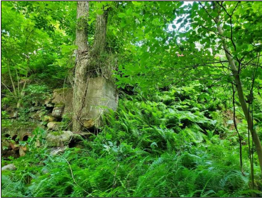
Photo No. 19. Downstream slope at STA 1+75 looking upstream. Note the deterioration of the dry set stone masonry LLO outlet headwall and the tree growing through the headwall.
