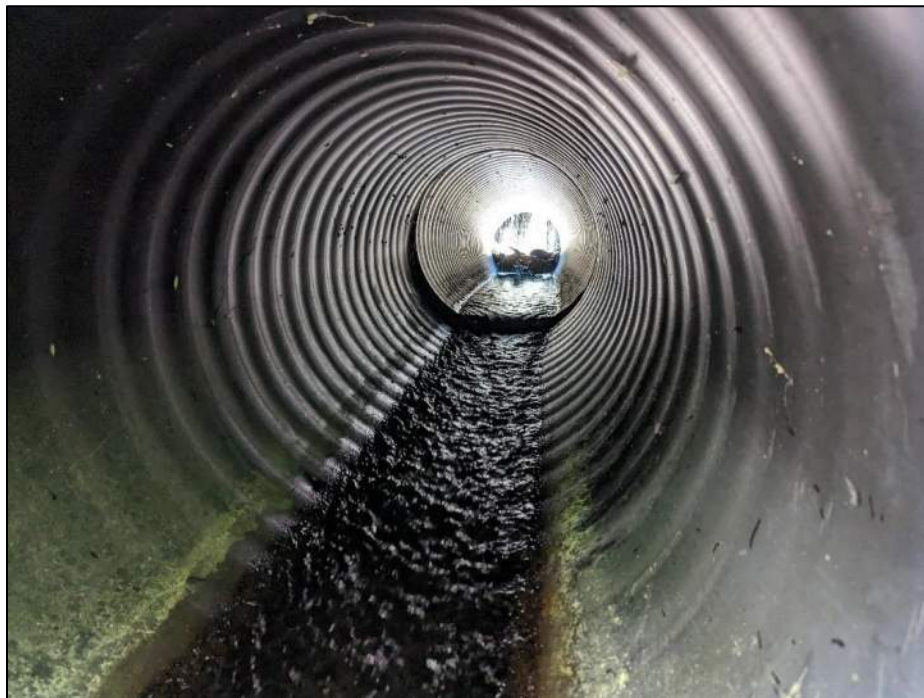
Photo No. 24. Interior of the left outlet pipe. Note the pipe is clear of debris, except for the entrance. Also note the displacement at the pipe joint midway up the pipe.
