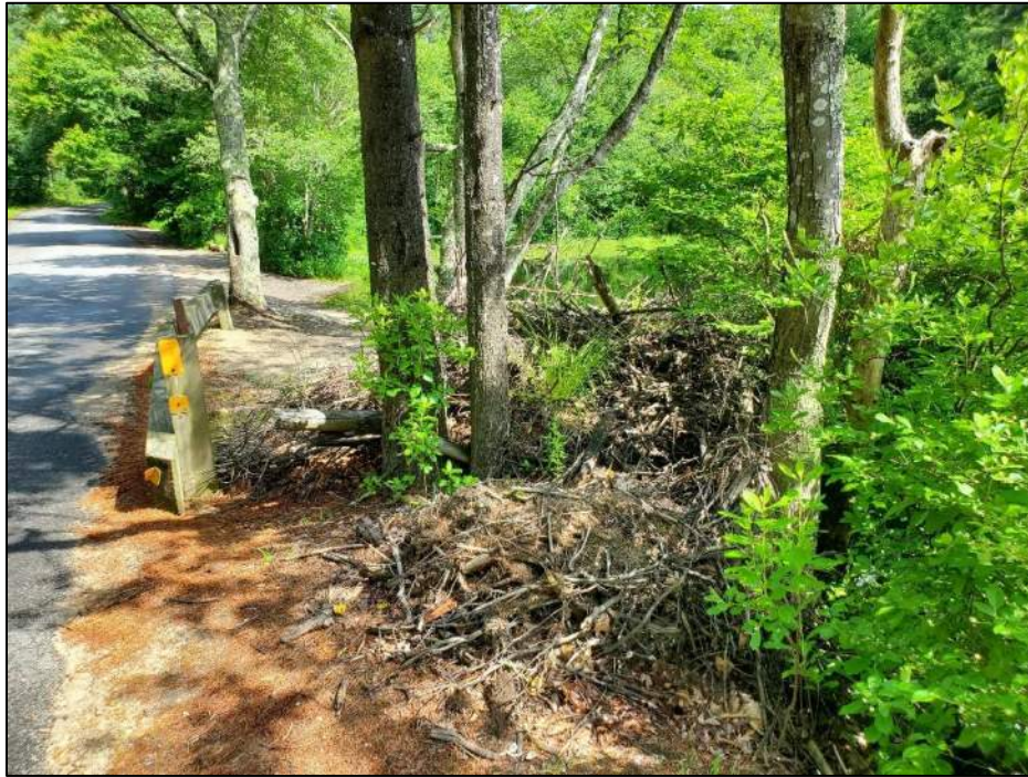
Photo No. 3. Upstream shoulder from STA 1+50 looking right. Note the trees up to 16 inches in diameter growing through the upstream slope and the pile of debris adjacent to the spillway.
