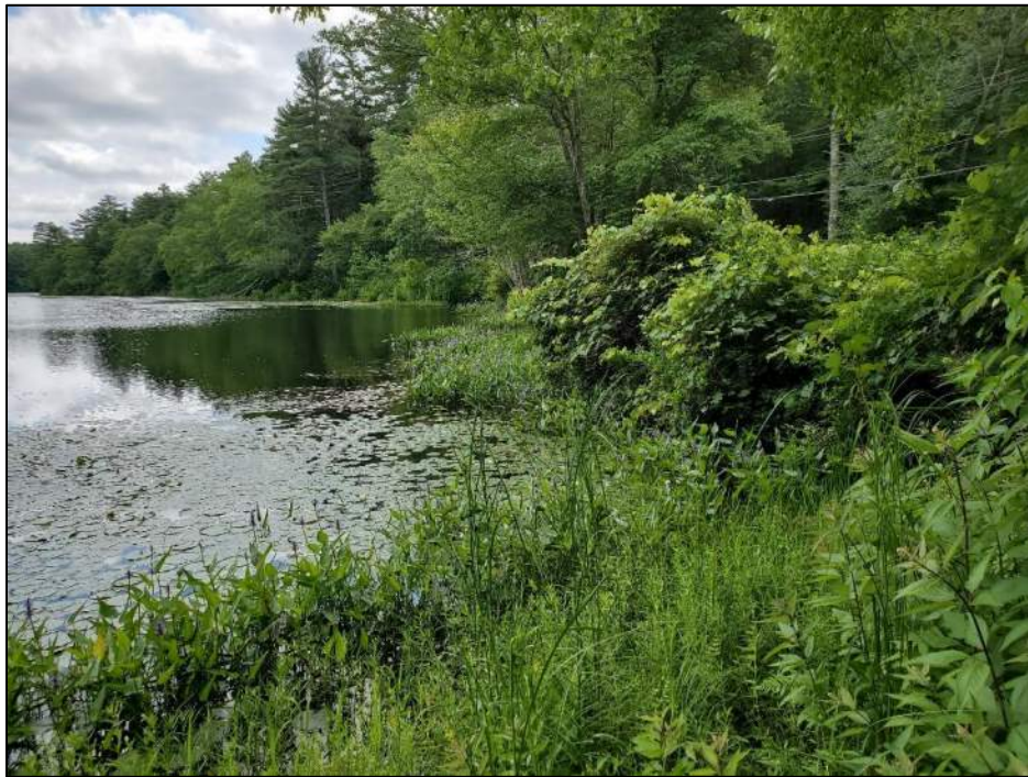
Photo No. 7. Upstream slope from STA 3+25 looking left. Note the dense woody brush and trees growing along the upstream slope.
