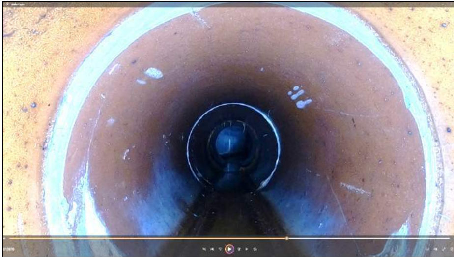
Photo No. 27. Interior of the vitrified clay LLO pipe approximately 40 feet upstream of the outlet as viewed during the conduit inspection. Note the apparent blockage at the end of the pipe.
