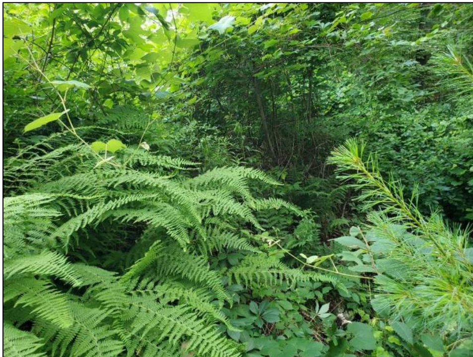
Photo No. 16. Downstream slope at STA 1+95 looking right. Note the dense vegetation and woody brush.
