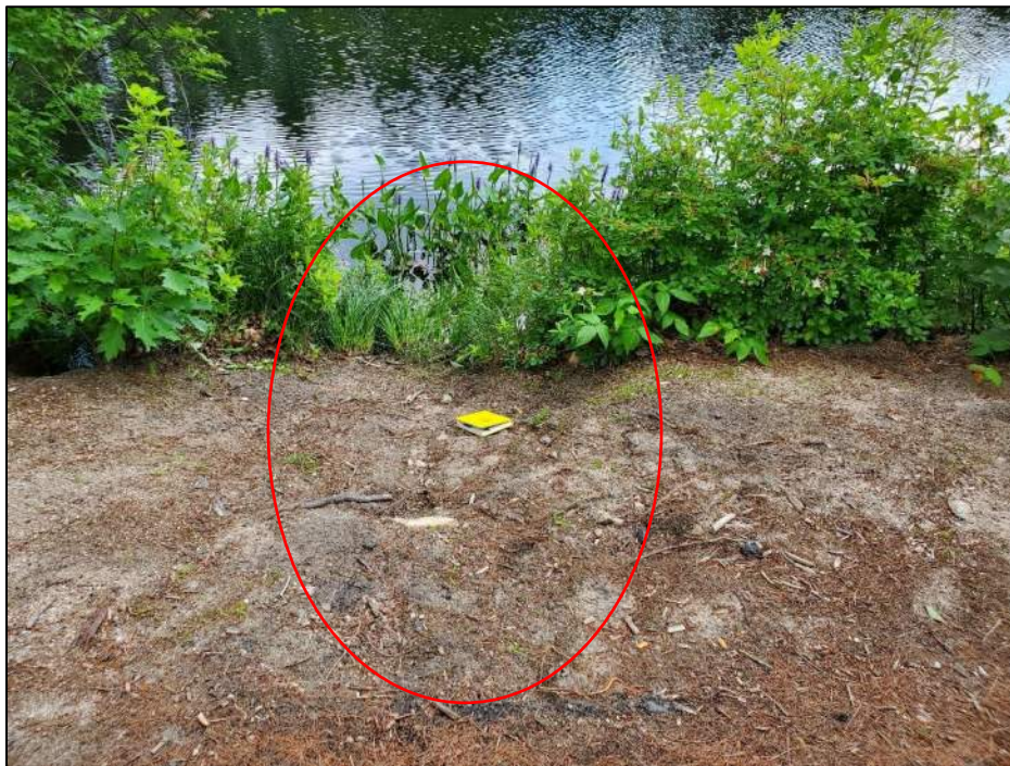
Photo No. 2. Upstream slope at STA 1+32. Note the erosion channel extending from Hopkins Hill Rd to Tarbox Pond (circle).
