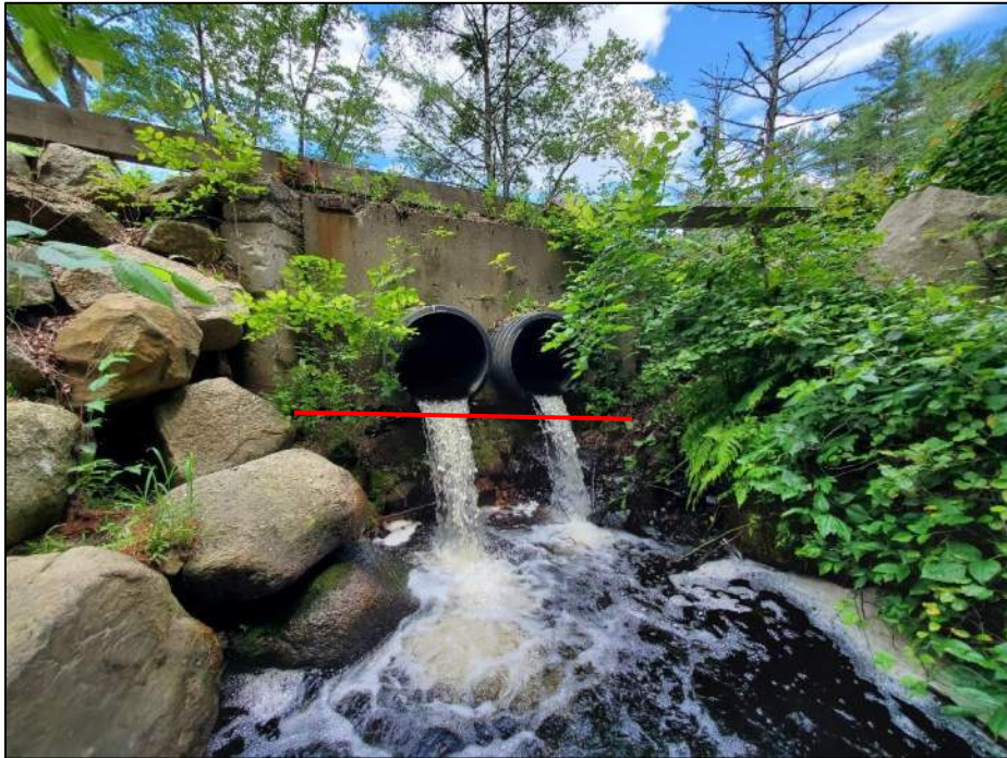
Photo No. 23. Spillway culvert outlets. The red line indicates the bottom of the concrete headwall. Below this elevation the headwall is partially supported by stone, but is beginning to undermine.
