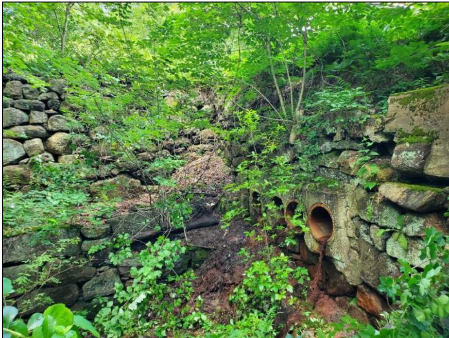
Photo No. 26. Historic LLO outlet structure. Note the woody brush growing through the headwall and downstream channel walls.
