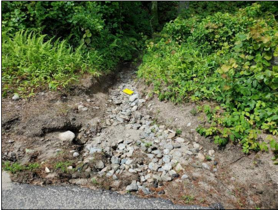
Photo No. 13. Downstream slope at STA 1+32. Note the erosion channel extending from Hopkins Hill Rd to Carr River.
