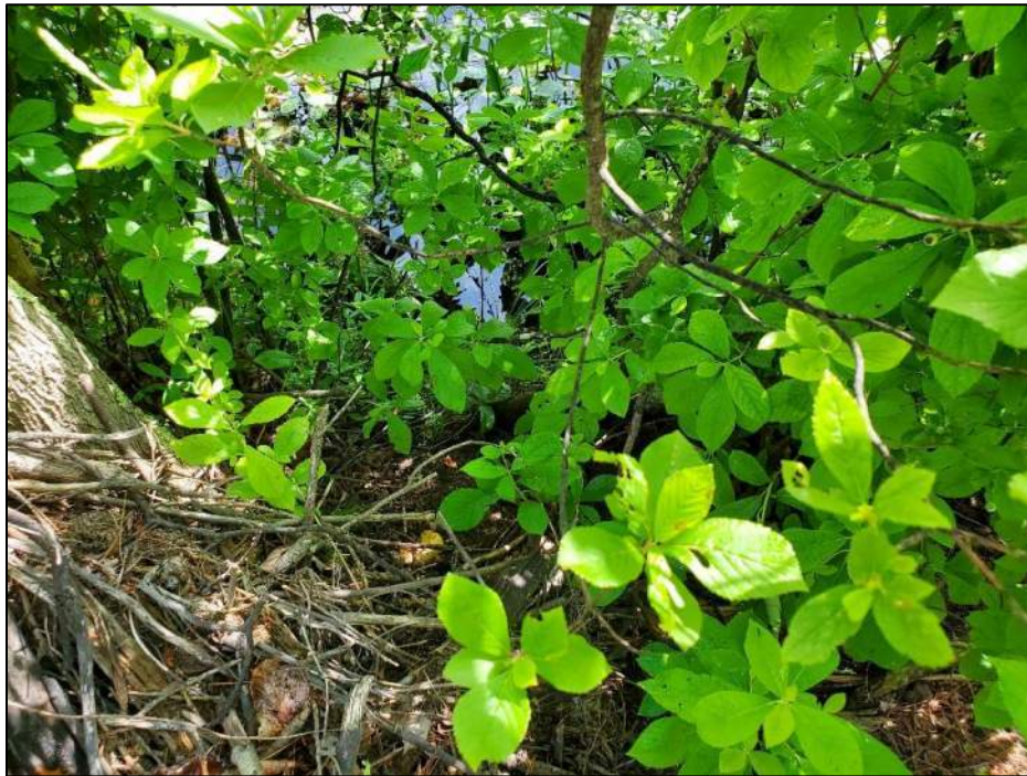
Photo No. 4. Upstream slope looking upstream at STA 1+50. Note the vertical scarping and dense woody vegetation.
