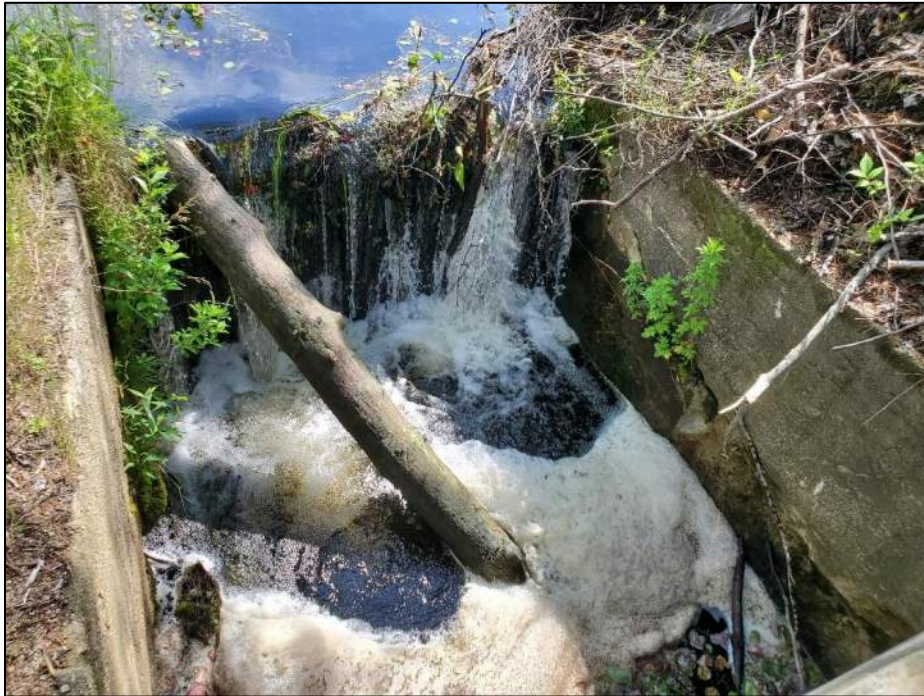
Photo No. 21. Spillway and stilling basin. Note the vegetation choking the spillway weir.
