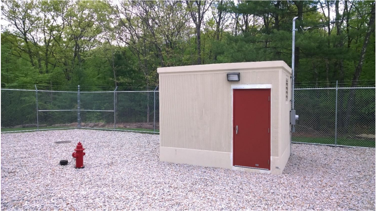
(Valve Station and Interconnect Building at Burlingame Site)
